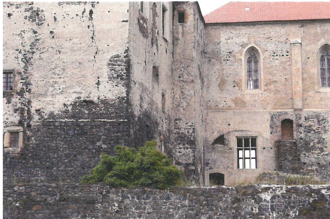
Fig. 21 (Right) Facades of Švihov Castle palace (left) and chapel (right), both from the late 15th century. The renders of the chapel were consolidated with limewater and conserved with lime-based materials in 2006, while the palace renders are still waiting. This makes it possible to compare the appearances of these precious facades before and after the conservation intervention. (G. Čapková, 2016)
