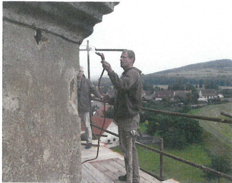
Fig. 13 (Above) Limewater is sprayed from a hose with a water spray nozzle. (Photo D. Michoinová)
